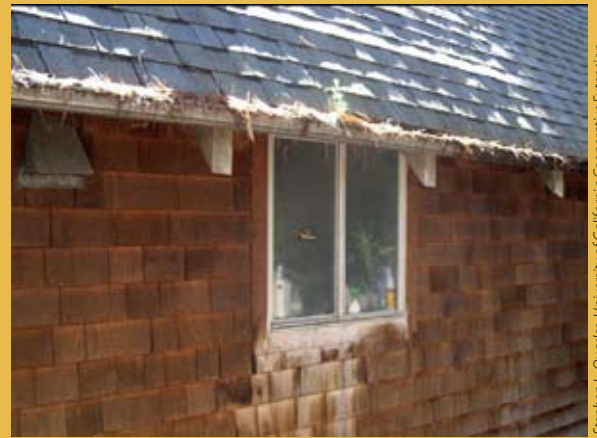
Accumulated fuel in rain gutter.
